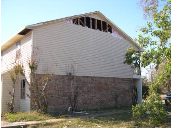
Figure 6. Failure of foam sheathing due to wind pressure (Hurricane Katrina, 2005).
