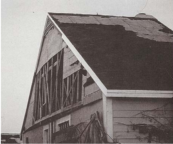
Figure 4. Failure of wood structural panel sheathing due to wind pressure (Hurricane Andrew, 1992).
