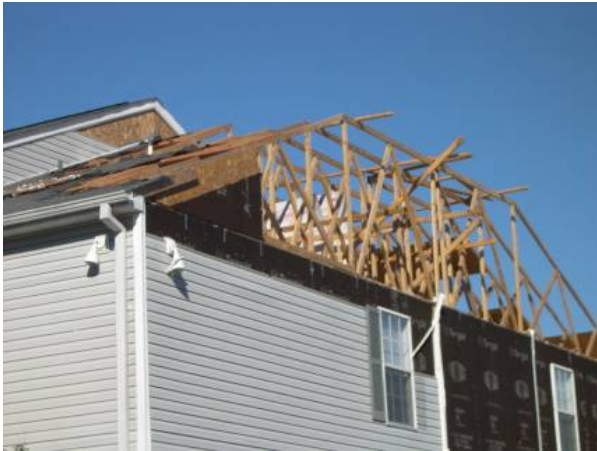
Figure 5. Failure of fiberboard sheathing due to wind pressure (Hurricane Katrina, 2005).
