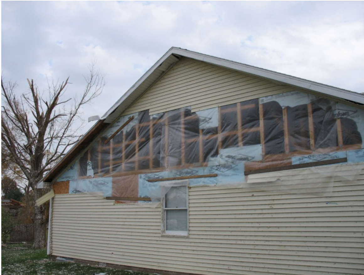
Figure 1. – Foam and vinyl wall covering failure. (Storm damage – Southern IN, 2005)
