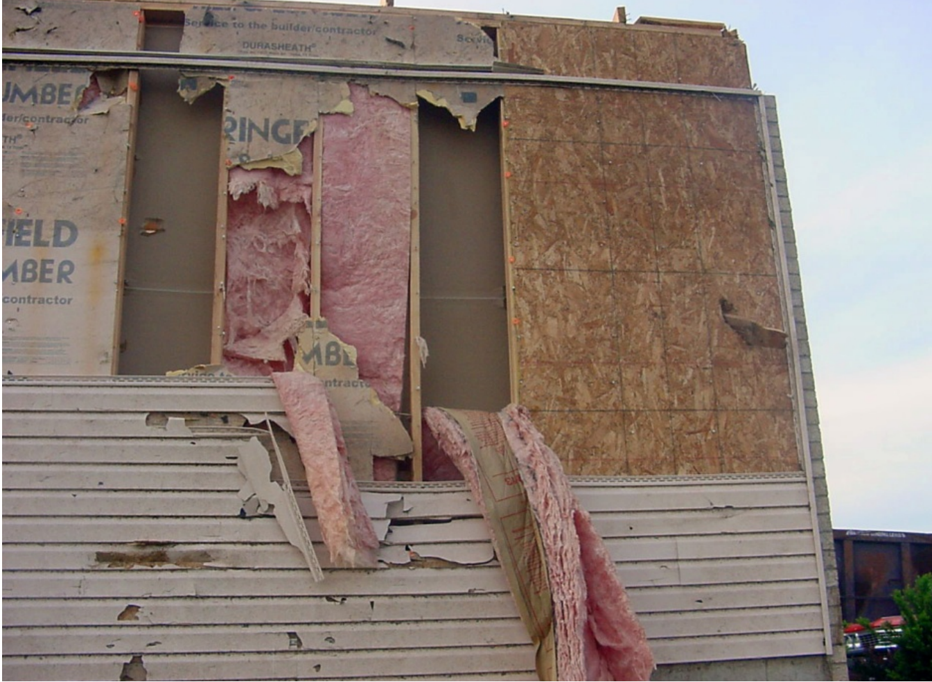
Figure 2. – Foam and vinyl wall covering failure while wall bracing panel remains. (Storm damage, Springfield, MO, 2006)
